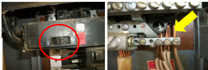
The breaker switch is
