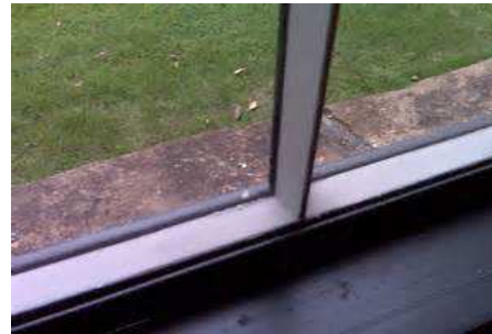
Cracked glass pane
